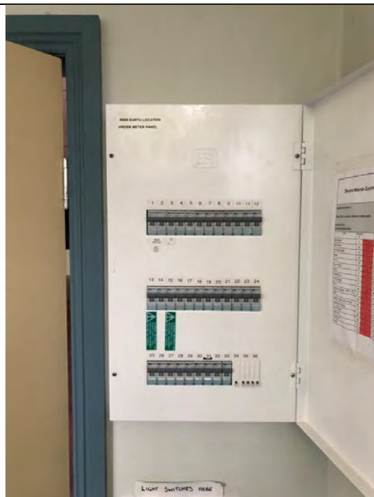
Figure 18- MSB located in Community Hall
