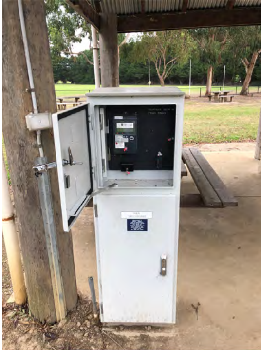
Figure 2- Authority meter panel installed in 2021 located in picnic shelter in Reserve
