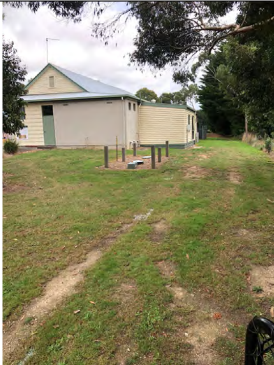
Figure 11- Onsite wastewater treatment plant located in NE corner of site
