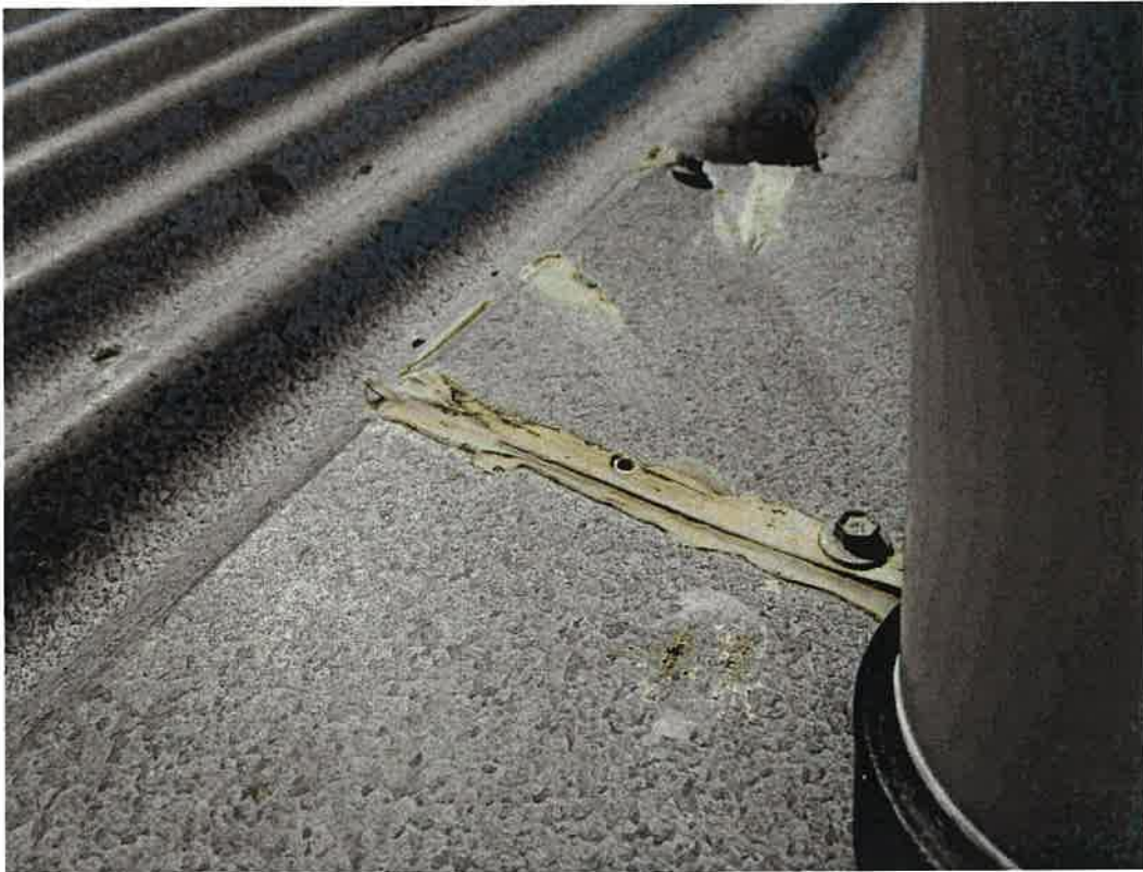
Photo 11; Example of poorly installed flashing. Missing roof screw and no pop rivets to hold sections together. Flashing not wide enough to extend to next corrugation fully. Screw at top not into top of corrugation.
