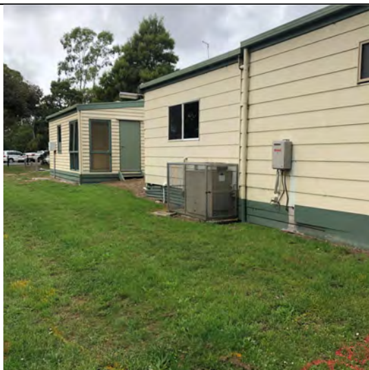
Figure 17- Gas heating furnace & DHW unit located on north façade
