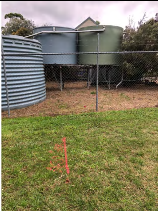
Figure 13- Onsite rainwater tank farm at rear of the site
