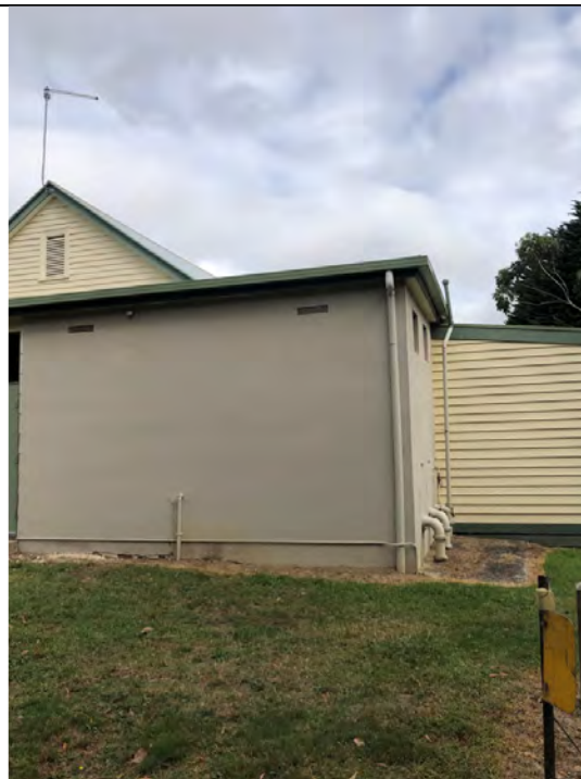
Figure 22- Sewer reticulation from local amenities adjacent the wastewater treatment system in NE corner of site
