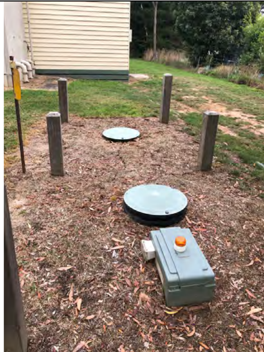
Figure 12- Wastewater treatment system with in ground storage/treatment tanks
