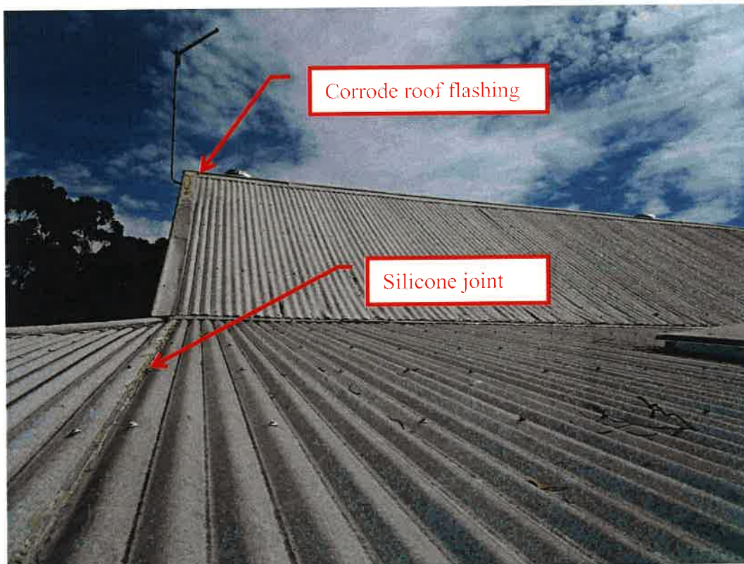
Photo 10; North side roof. Silicane joint. Corroded roof flashing.
