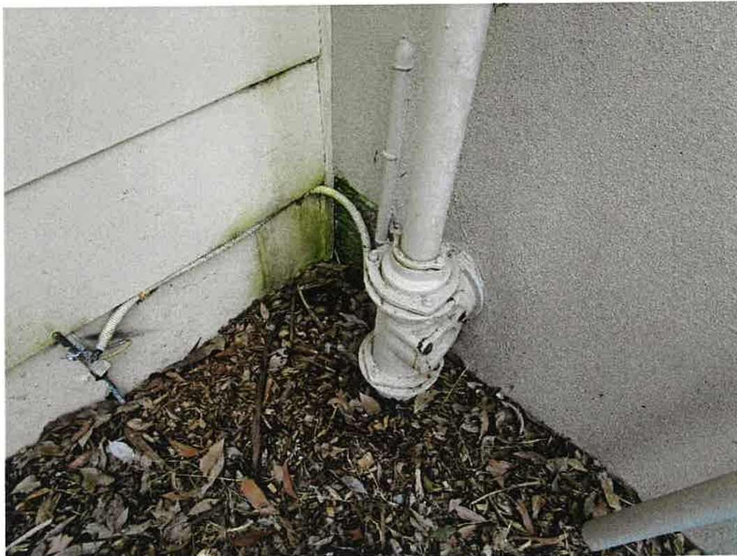
Photo 4; South east re-entrant corner. Algal growth indicating high moisture levels.
