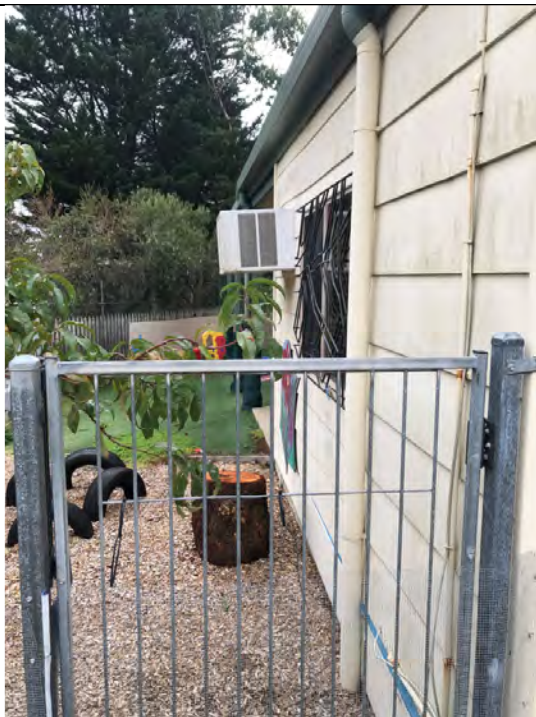
Figure 25- Room A/C unit located in childcare area at rear of the facility
