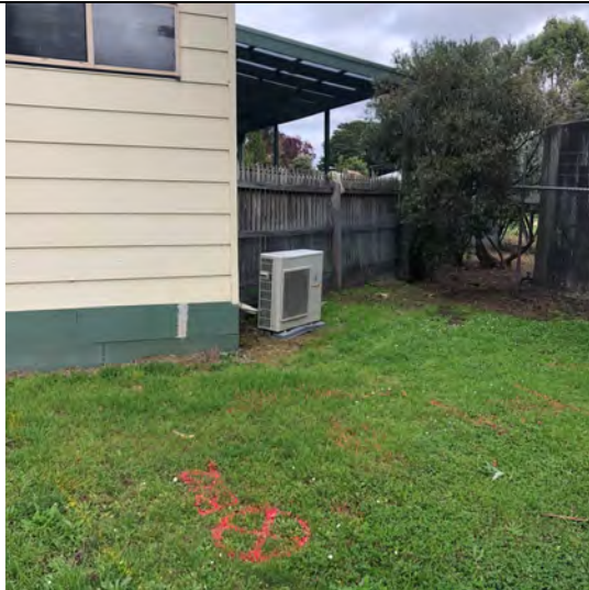
Figure 23- Condenser unit located on ground at rear of the building
