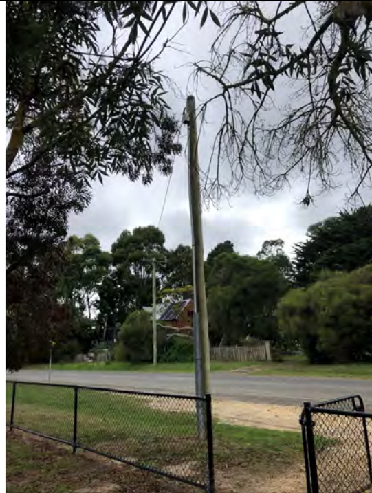
Figure 3- Existing overhead supply to the Reserve MSB/meter panel
