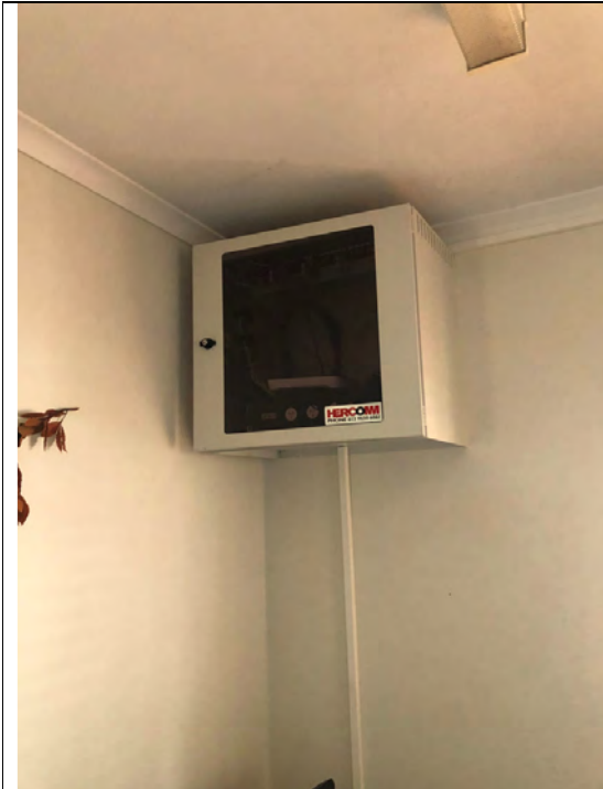
Figure 9- Comms rack located in MCH area of Community facility
