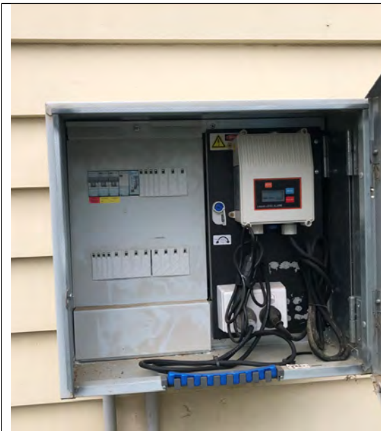
Figure 21- Wastewater Treatment system control panel
