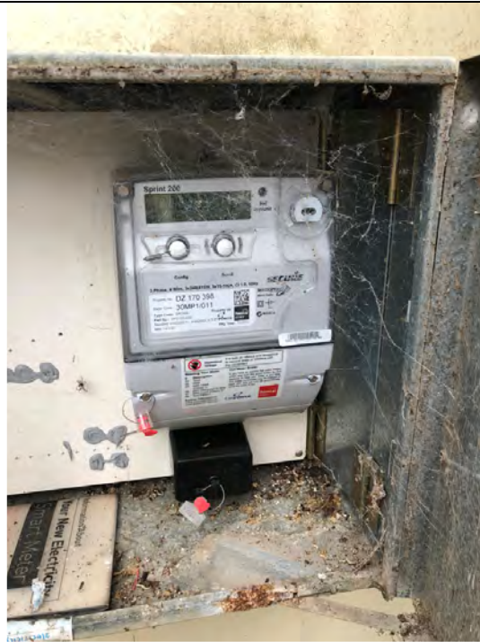
Figure 7- Existing meter panel located on the Community Hall facility
