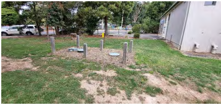
Site conditions – Photo showing the wastewater treatment system
