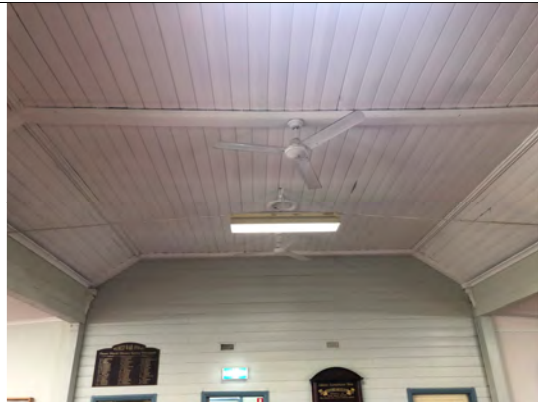
Figure 19- Existing lighting & ceiling fan in community hall
