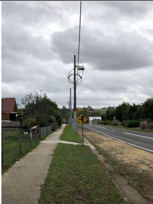
Figure 6- Nearest overhead HV service on Winchelsea-Deans Marsh Road
