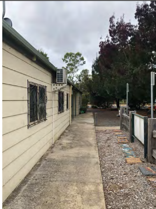
Figure 24- Condensing unit located on façade bracket at high level, installed in 2021
