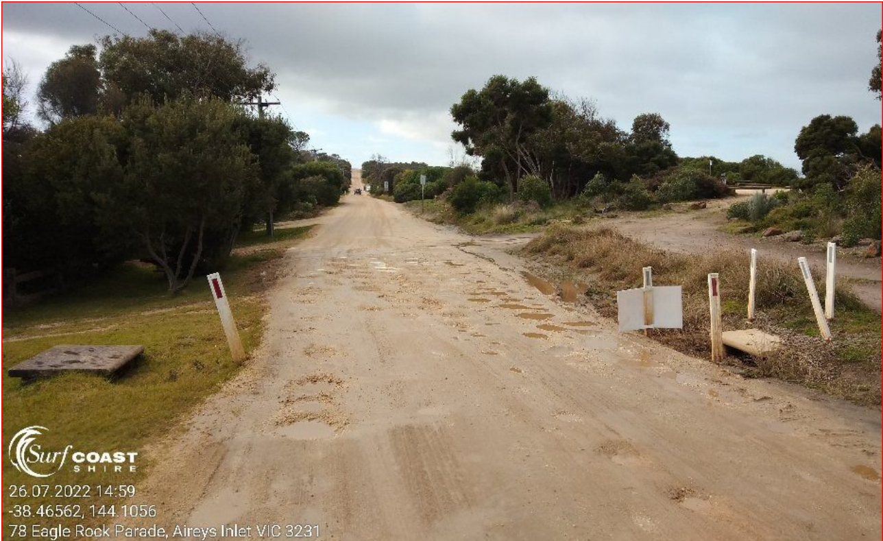
Figure 1: Unsealed Road Pothole Damage (Source: Courtesy Surf Coast Shire)
