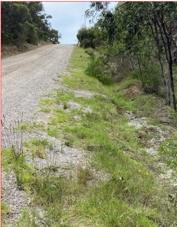
Figure 19: Boundary Road, Aireys Inlet - steep hill with road rutting and erosion
