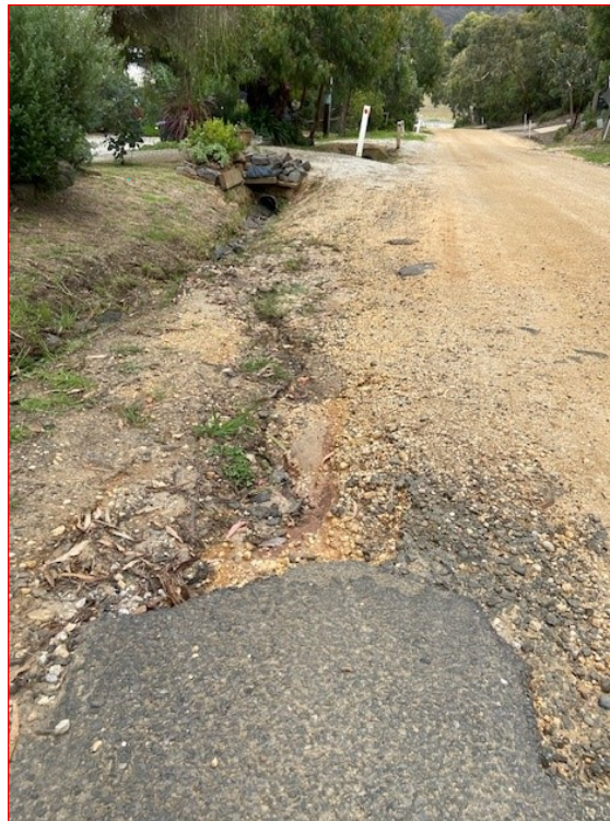
Figure 20: Aireys Street, Aireys Inlet- steep hill with washout erosion between sealed intersections
